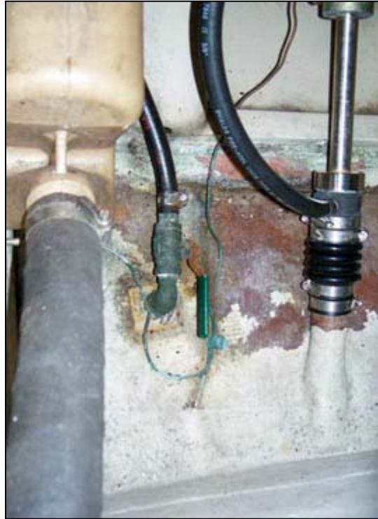
These three inadequate items must be replaced when repowering (left to right): a thin plastic muffler, an improper seacock installation with a ball valve, and a "dripless" stuffing box.
